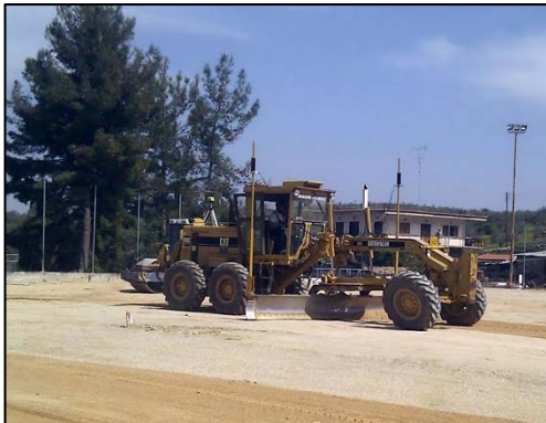
The grader managed the levelling of the whole sports field in only two hours
