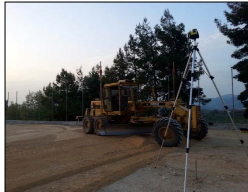
The laser signal from a dual slope laser transmitter served as height reference for the levelling system
